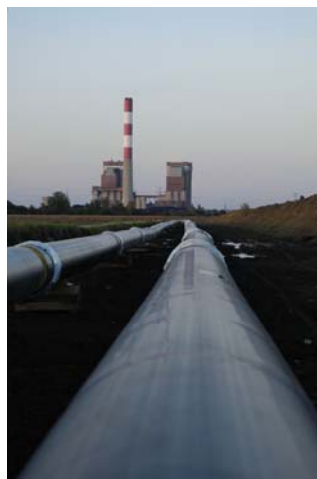
Pipeline. Foto: UlrichUlrich, CC BY-SA 3.0
